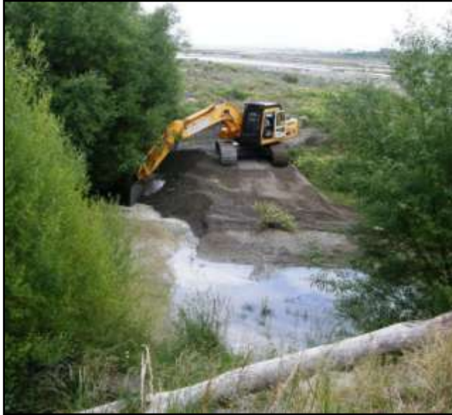
Taggart's digger excavating a swimming hole off the end of Groyne 1 just before Christmas, 2011.
